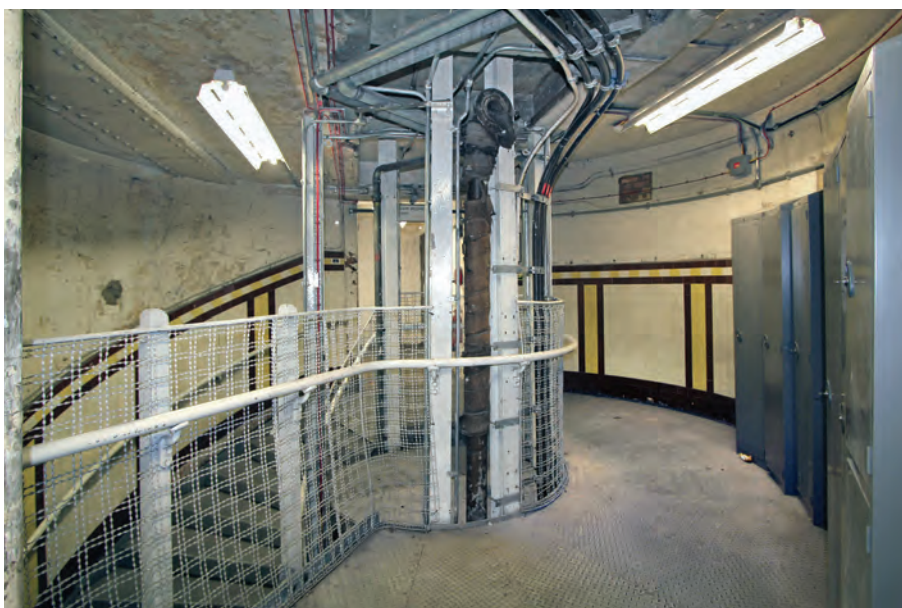
The top of the emergency stairs. The stairs have been replaced but the distinctive wall tiling which is unique to Hyde Park Corner remains in good condition.
